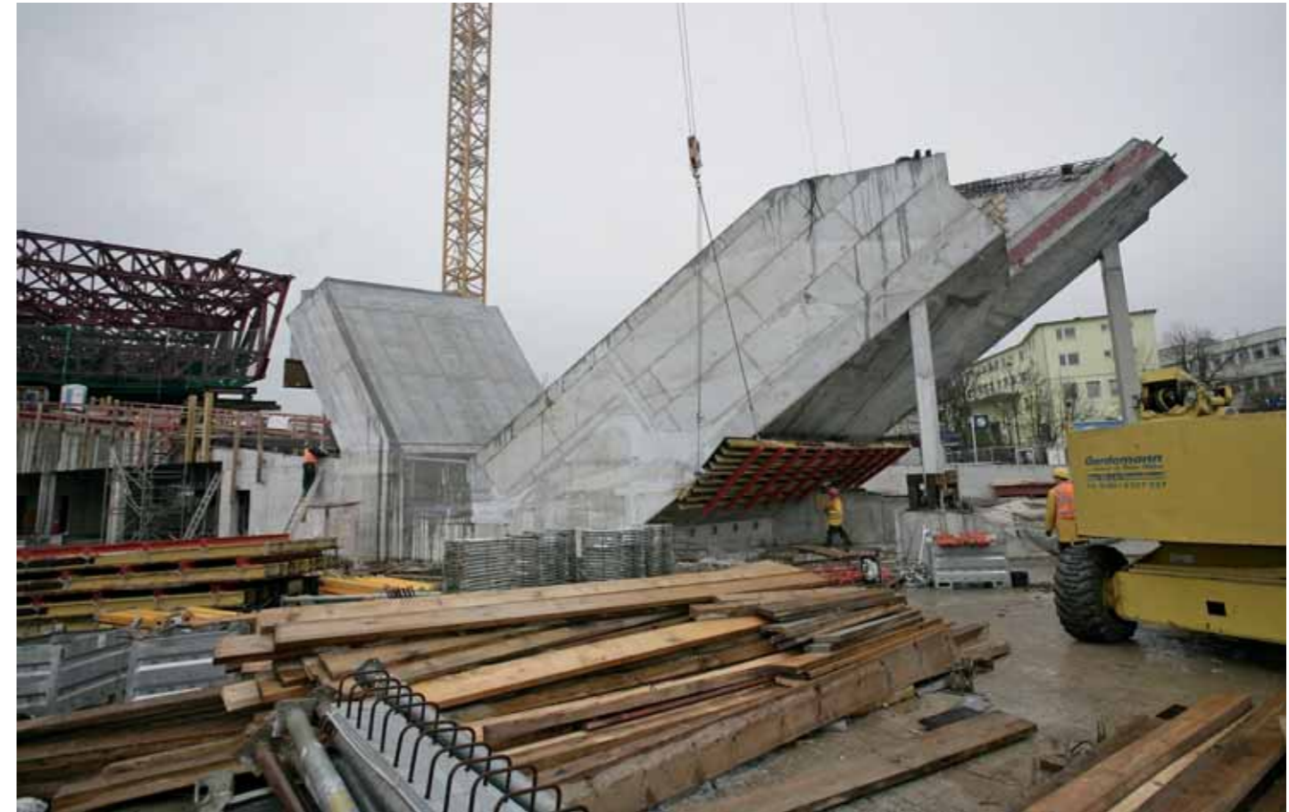
Supported: One of the concrete cores that are to carry the bold steel structure is shaped like a “lying Y”
